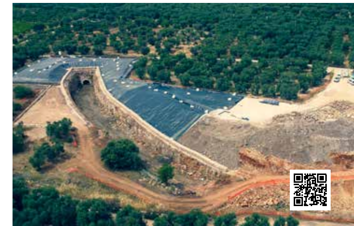
Sannicandro (BA), remediation and permanent safety measures for the former municipal landfill
