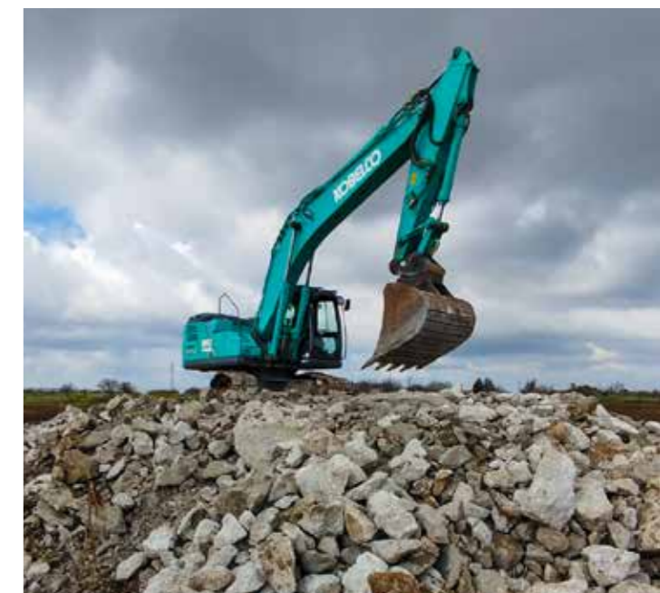
Municipality of Melissano (LE), foundation slab demolition works at the former photovoltaic plant
