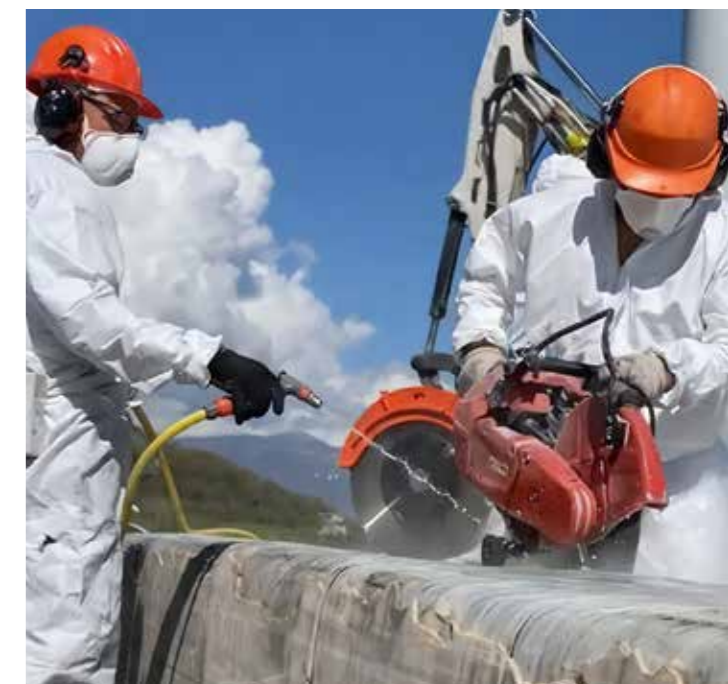
Municipality of Campagna (SA), interventions at the wind farm for volume reduction and plastic waste management
