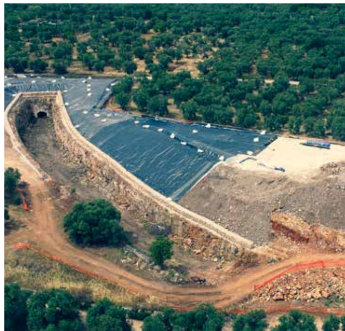
Sannicandro (BA), Remediation and Permanent Safety Measures for the Former Municipal Landfill
